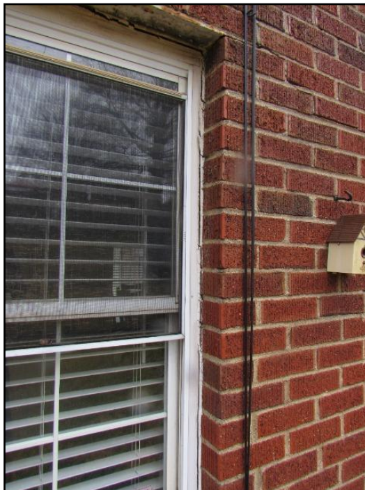
12. Caulking loose, missing or deteriorated
