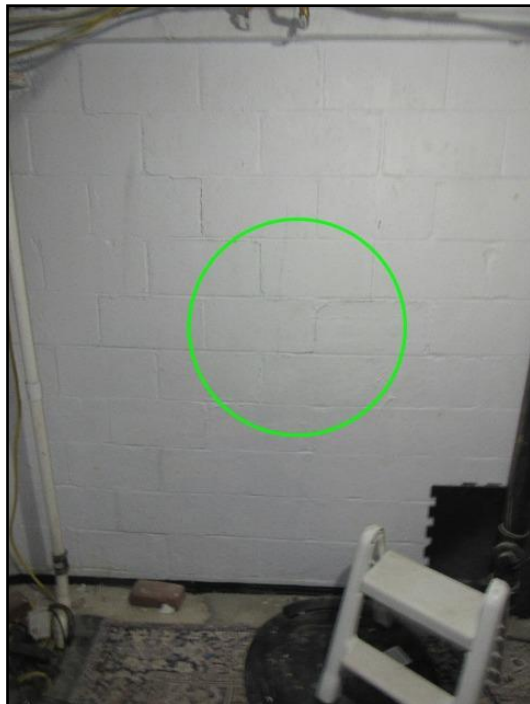
22. Bowed, bulging or leaning
