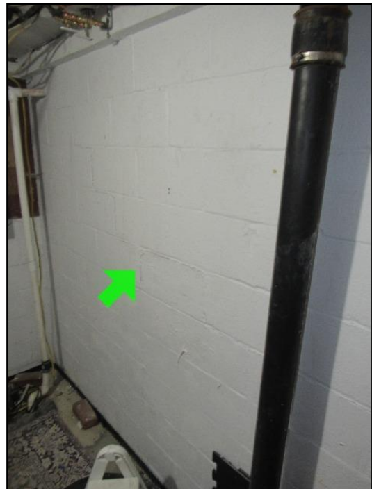
23. Bowed, bulging or leaning
