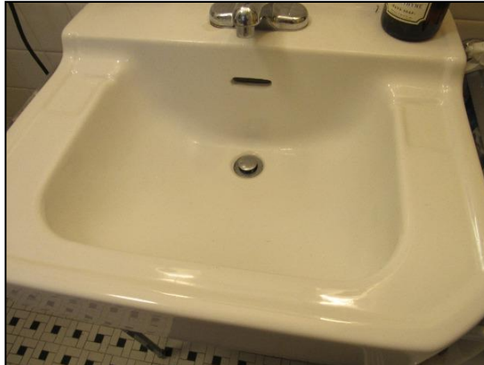
39. Drain stop ineffective
