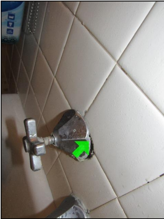
40. Caulking loose, missing or deteriorated
