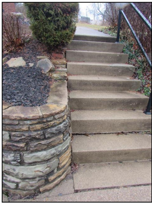
17. Steps or landings settling or heaving
