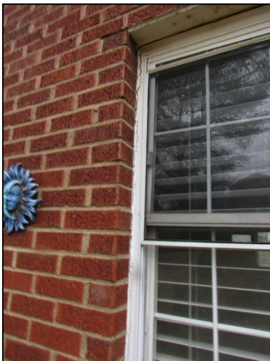
10. Caulking loose, missing or deteriorated
