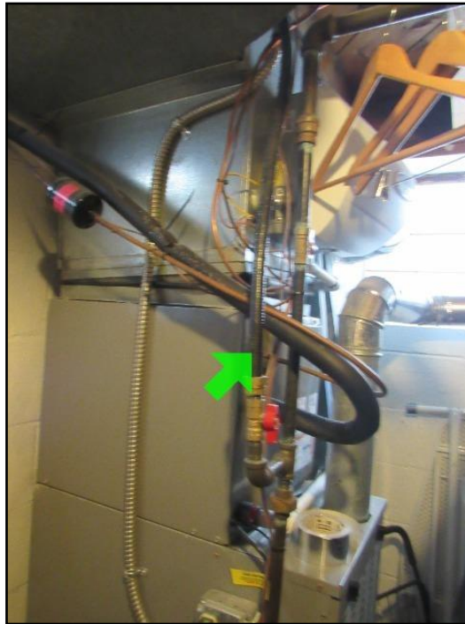
37. Piping not properly bonded
