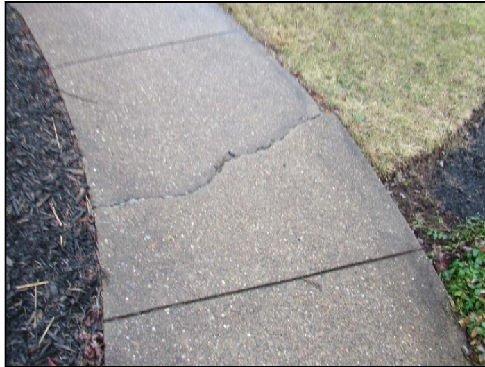
18. Cracked or damaged surfaces
