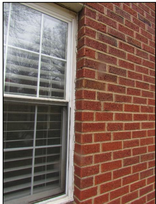
11. Caulking loose, missing or deteriorated
